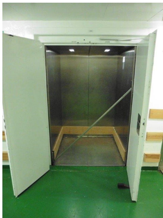
Goods lift (main deck level) open
