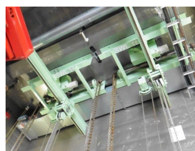
Winch above shafts
